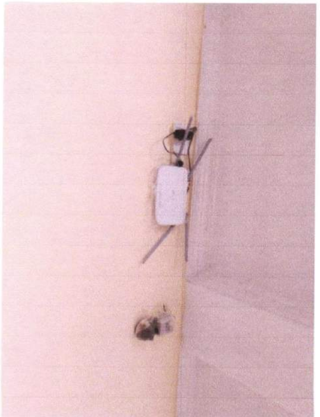
Wifi Router Third Floor 2
