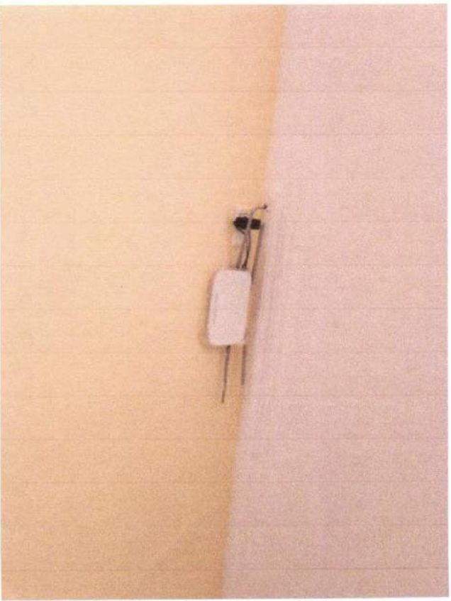
Wifi Router 5th Floor 1
