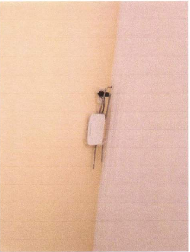
Wifi Router 4th Floor 2
